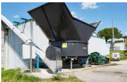
Open transfer to existing conveyor system
