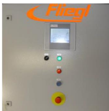
Fig. 7: Small control cabinet
