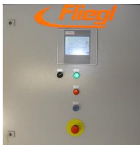
Fig. 2: Small control cabinet
